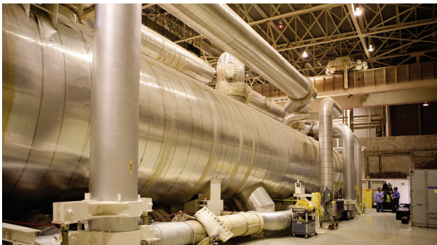
Columbia Generating Station
