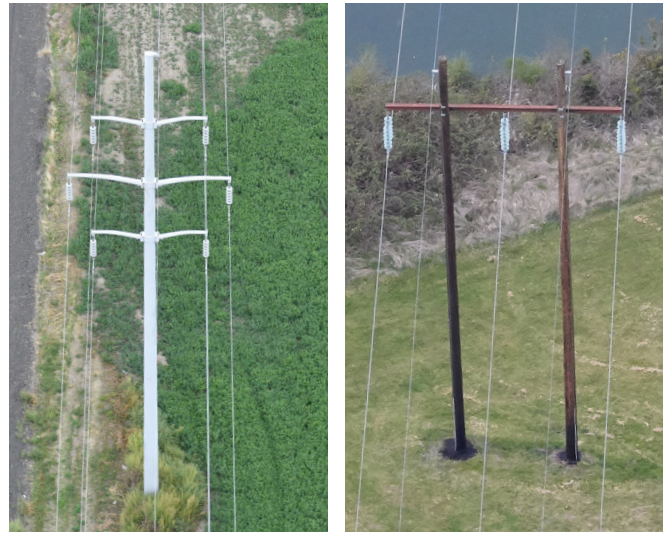
(LEFT) Double-circuit steel pole structure (RIGHT) H-frame wood pole structure
