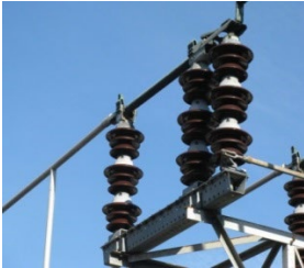
115 kV Disconnect Support
