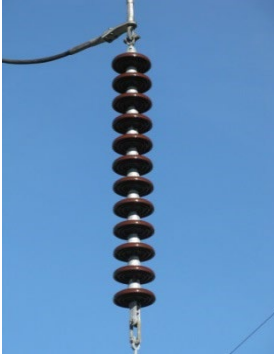
230 kV Riser Bus in Bridge
