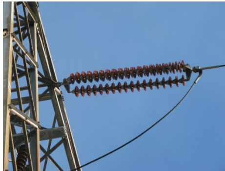
230 kV Line Dead End
