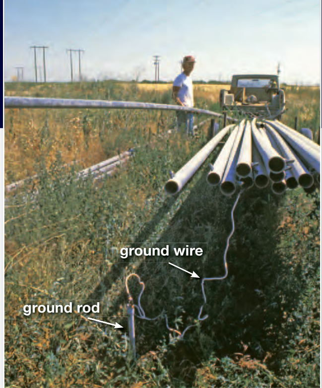
The possibility of nuisance shocks can be eliminated by grounding metal pipe when unloading near BPA lines.
