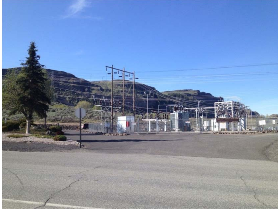
Figure 3-22. View of the Grant County PUD Substation and Transmission Line from the Grand Coulee Middle School
