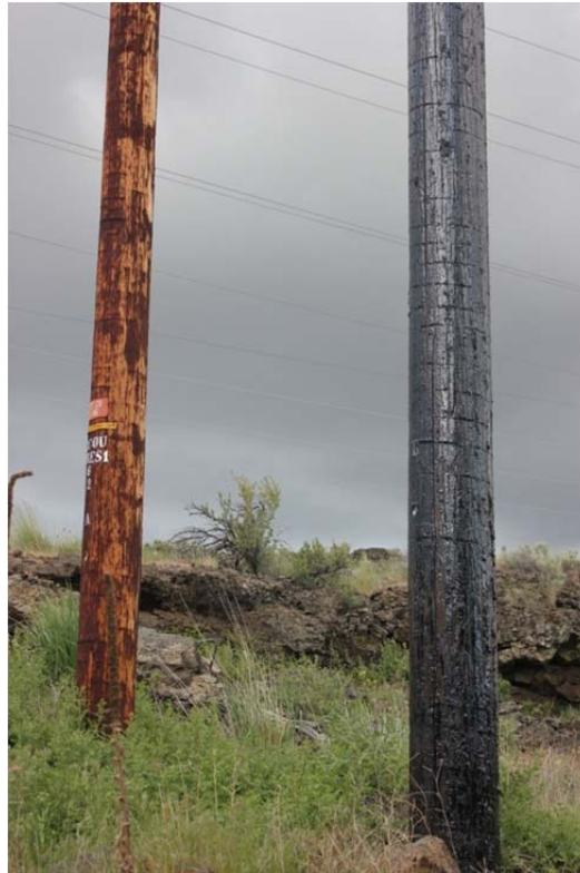
Figure 1-2. Example of Structures in Poor Condition
