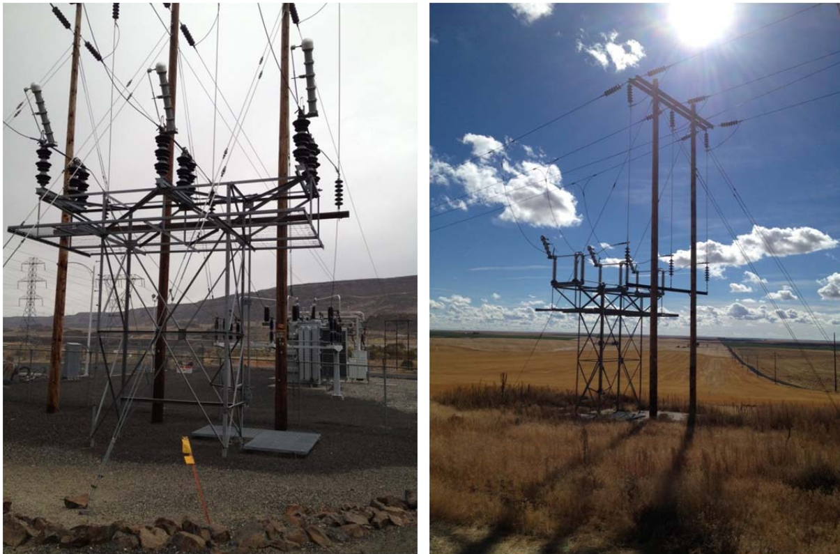
Figure 2-3. Grant County PUD Tap on Left, Wilbur Tap on Right
