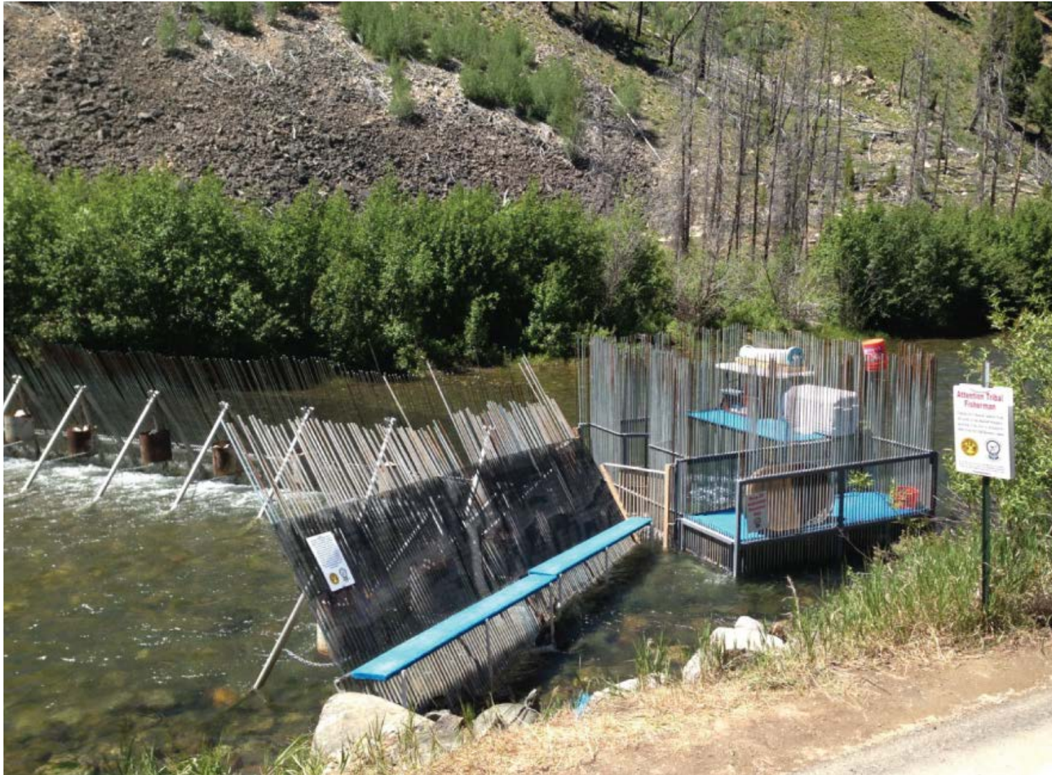
Figure 2-11. Example of a Temporary Weir Structure Proposed at the Yankee Fork and Panther Creek Weir Facilities under Alternative 2
