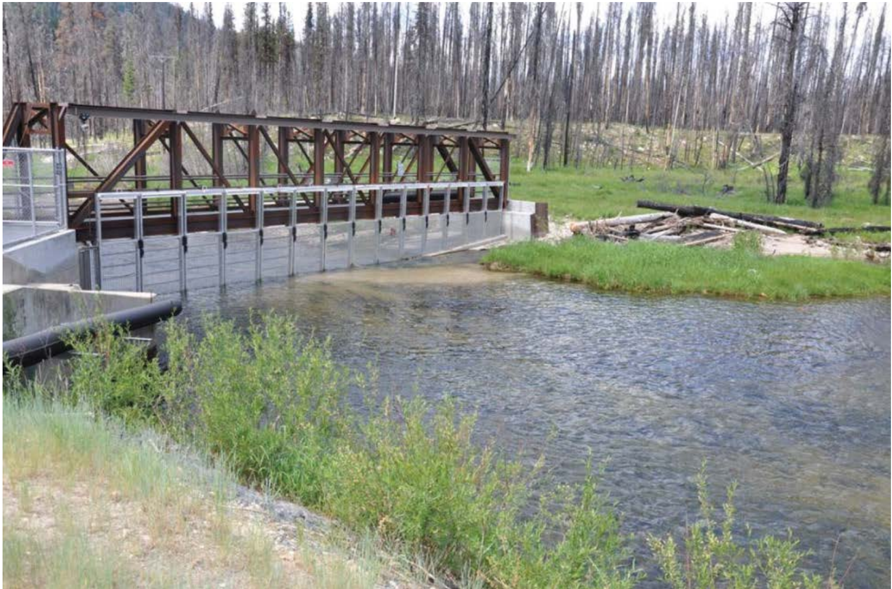
Figure 2-6b. Example of Bridge Weir in Operation (South Fork Salmon River Bridge Weir)
