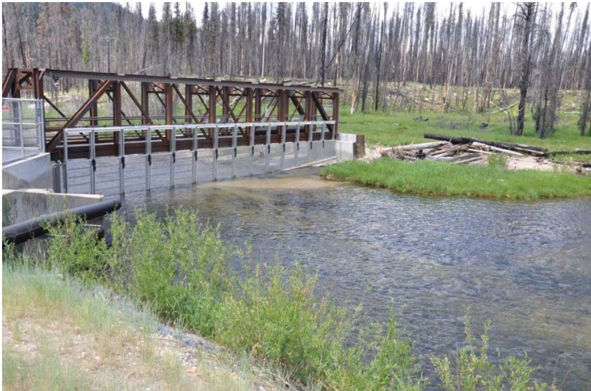
Figure 8. Example of a bridge weir in operation
