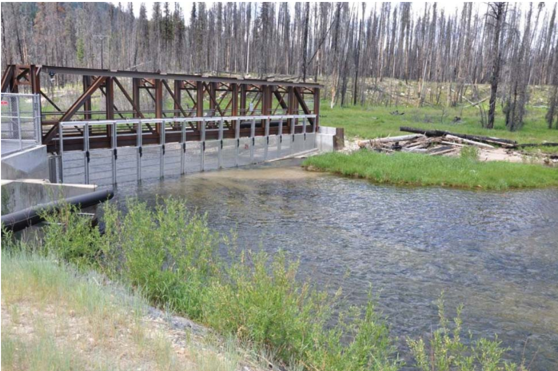
Figure 10. Example of a bridge weir in operation
