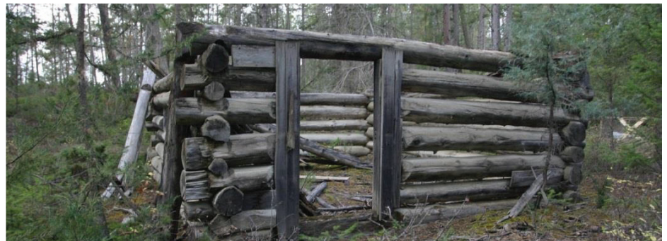
Historic log cabin located during an inventory survey at Lake Koocanusa, Libby, MT, FY 2015.
