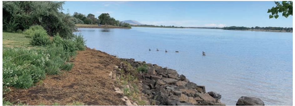
1,000-meter long bank stabilization of a large pre-contact village site at the McNary Project to protect it from erosion and recreational impacts, FY 2019.
