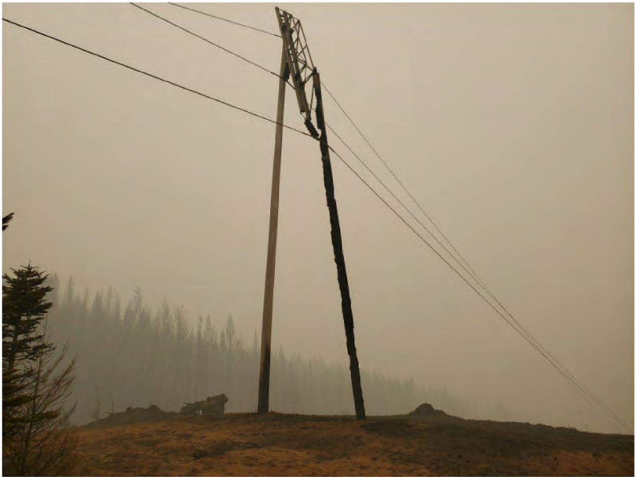
23/3 A pole okay, B pole some fire damage, it can wait for now. C pole REPLACE, its gone. Conductor on the ground, no Conductor damage. See attached picture
