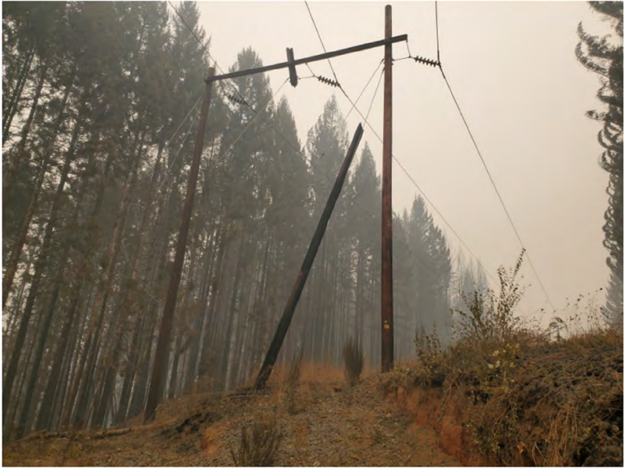
16/4, A pole good, REPLACE B pole, see picture below.
