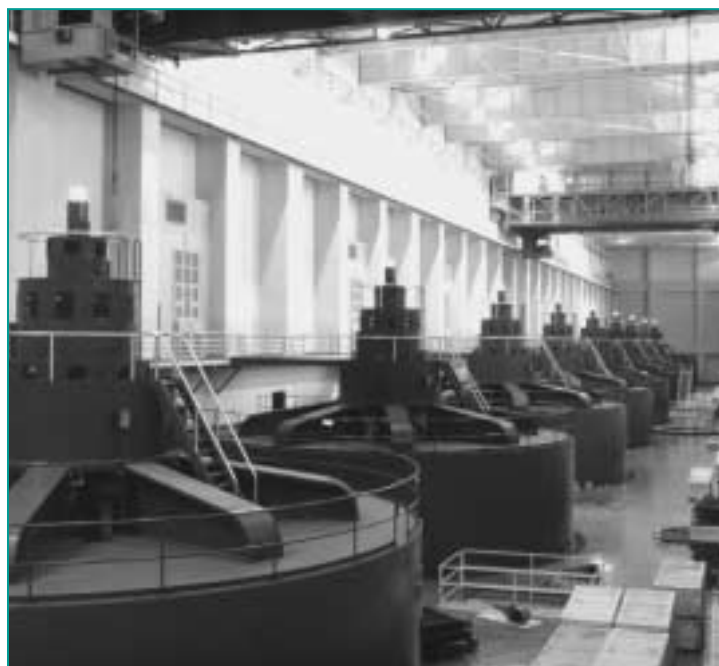
Coordination allows generators to plan routine maintenance at individual plants, such as Bonneville Dam, without disrupting their ability to serve load.
