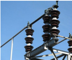
115 kV Disconnect Support
