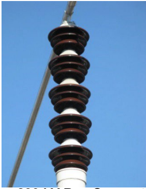
230 kV Bus Support
