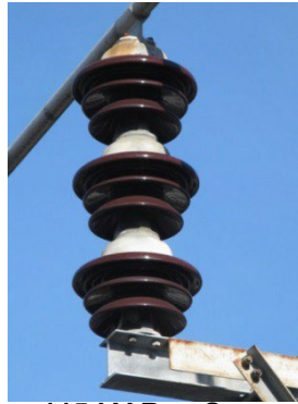
115 kV Bus Support
