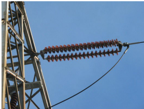
230 kV Line Dead End
