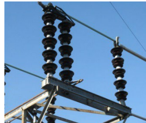
230 kV Disconnect Support
